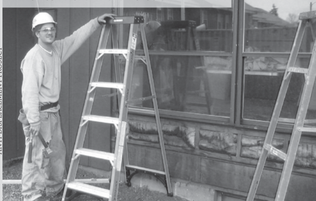
JOEL RODRIGUEZ, A-DP LEADER AND NEW MEMBER OF THE CARPENTERS LOCAL 108 WORKING ON UNION CONSTRUCTION JOB SITE AT CATHEDRAL HILL APARTMENTS, A-DP'S MOST RECENT TENANT BUYOUT.
